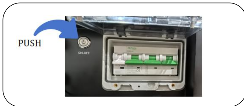
Figure 32 The Power Switch Of Battery Systems
