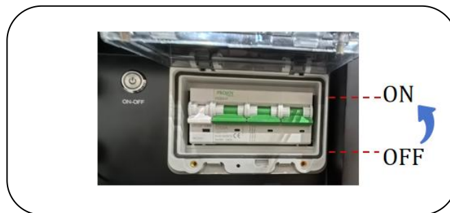
Figure 29 Open the Circuit Breaker on BDU
