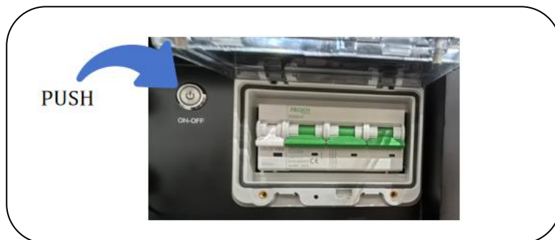
Figure 32 The Power Switch Of Battery Systems
