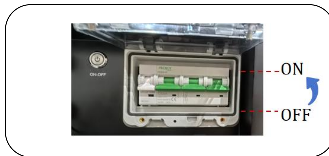
Figure 29 Open the Circuit Breaker on BDU
