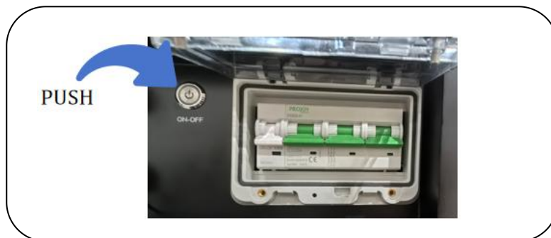
Figure 32 The Power Switch Of Battery Systems
